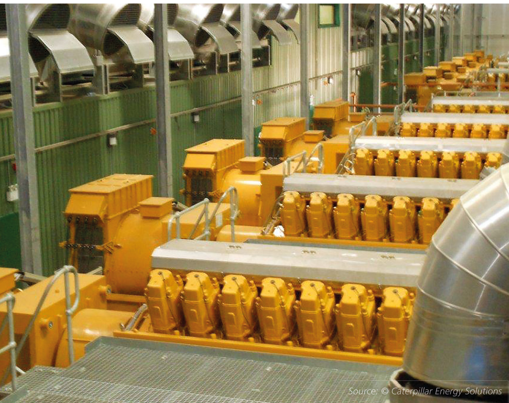
Gas engines for energy generation.
