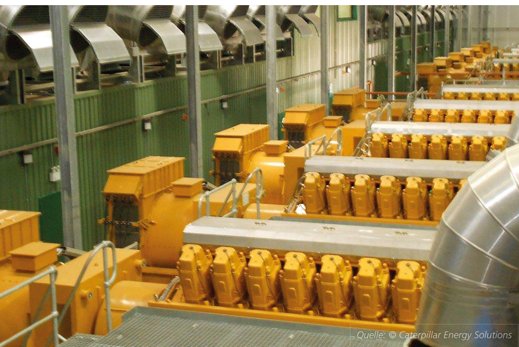
Gasaggregate zur Stromerzeugung.
