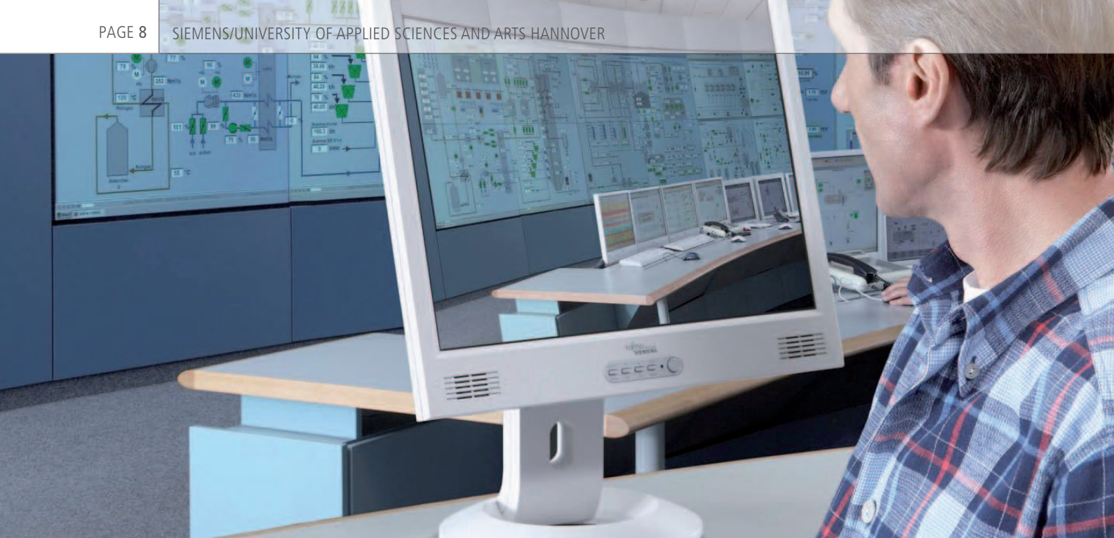
Figure 3: Large steam turbine power plants are automated with the T3000® turbine control system from Siemens AG.
